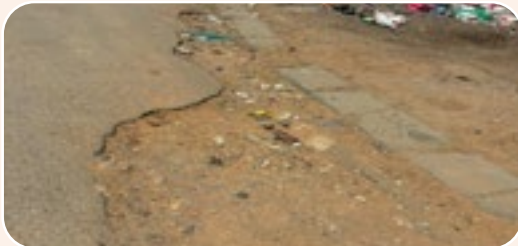
Pothole in September 2024
