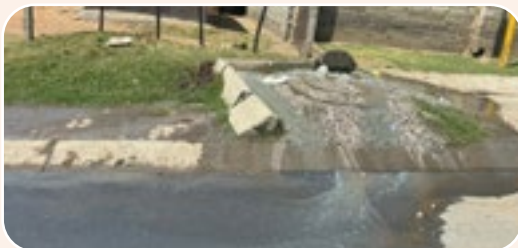
Sewage flowing onto the road
